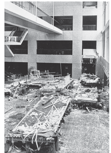
FIGURE 9–1 Elevated walkway collapse in a Kansas City hotel in 1981. How a simple physics calculation could have prevented the tragic loss of over 100 lives is considered in Example 9–12.
