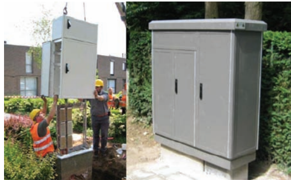
Figure 16. Replacement cabinet FTTC implementation
