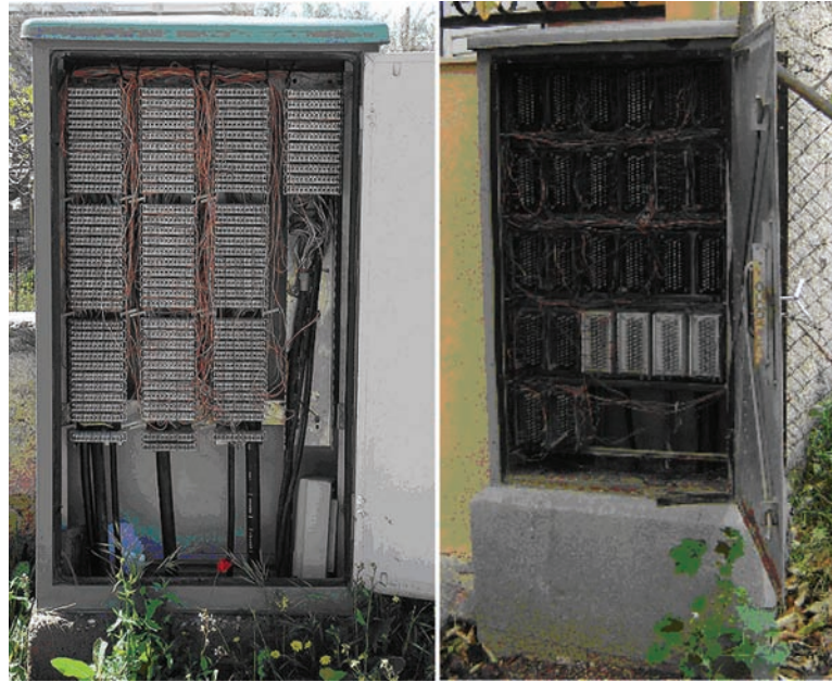
Figure 2. OTE XCC cabinets (new and old types) allowing for up to 1,200 and 750 pair terminations respectively. A primary to secondary cable pair ratio of 2:3 is used.
