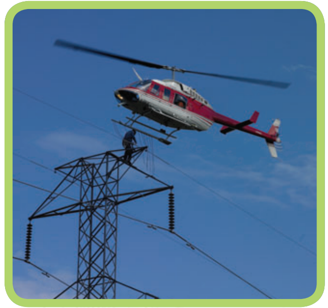
Transmission lineman performs maintenance work on a 240 kV transmission line with the assistance of a helicopter.
