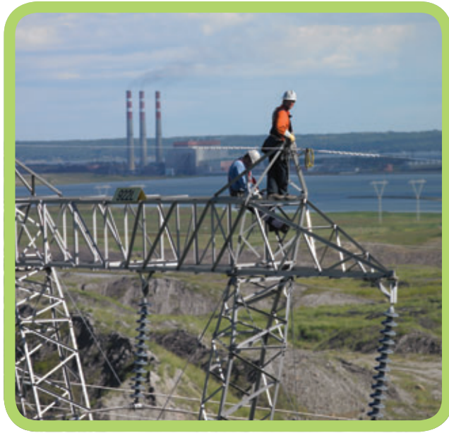
Ted Graham, North Transmission Line Crew Foreman, and Josh Krebbs, Transmission Lineman, perform maintenance work on a 240 kV transmission line. TransAlta's Sundance generation plant is in the background. Ted and Josh are retying the overhead protective shield wire. The overhead shield wire protects the transmission line from lightning damage.
