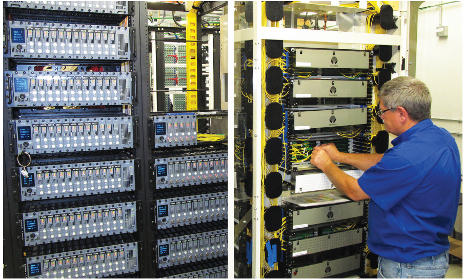
Cable, phone and Internet service originate at Country Cablevision's control site in Yancey County.
